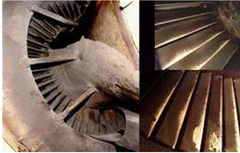
Figure 6-9 Fouled Compressor Inlet and Compressor Blades [40]
